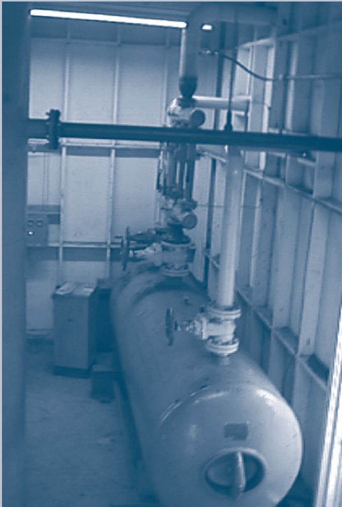
To stabilize system pressure, compressed air is stored in containers such as this 800-gallon horizontal unit.
