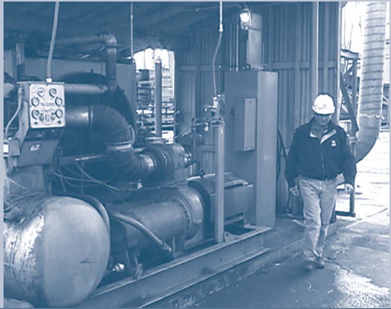
The largest of three rotary screw compressors at the mill is this 300-hp unit.
